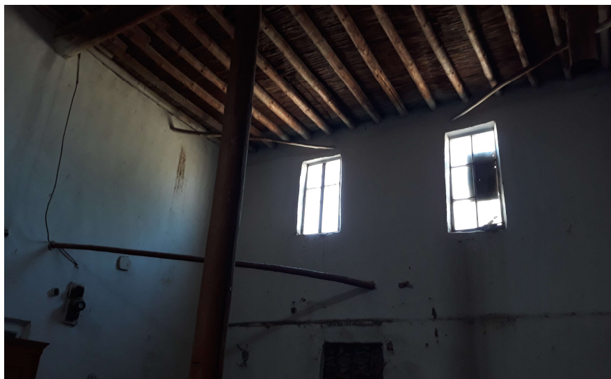
Figure 3. Interior view of old houses
